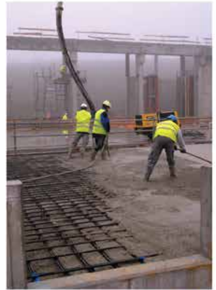
The first concrete is poured at ITER in 2010, inaugurating the facility's construction in earnest.
