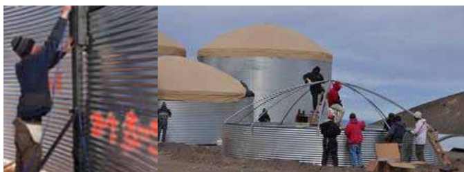
Figure 2. On the left, a custom jack-stand being installed by Patrick Younk. On the right, a work crew assembling the roof of the WCD structure.
