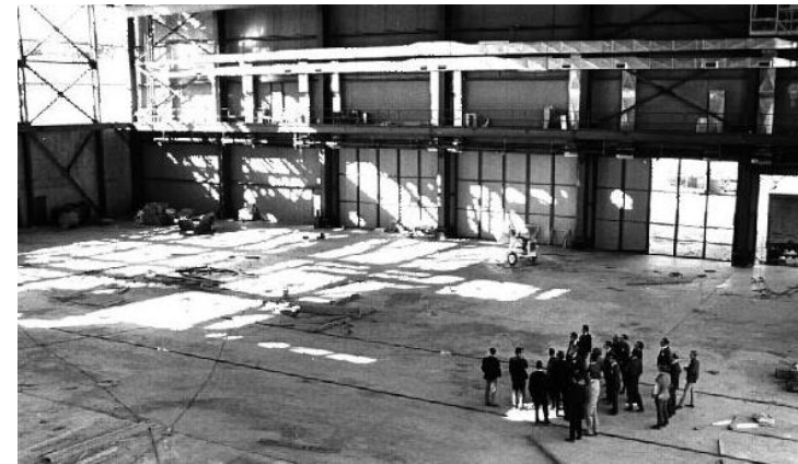
Area A is almost ready for the installation of beam equipment – in 1970 and now
