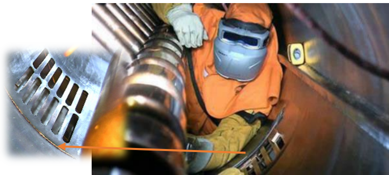
Failed weld inside drift tube linac caused significant loss of beam time
