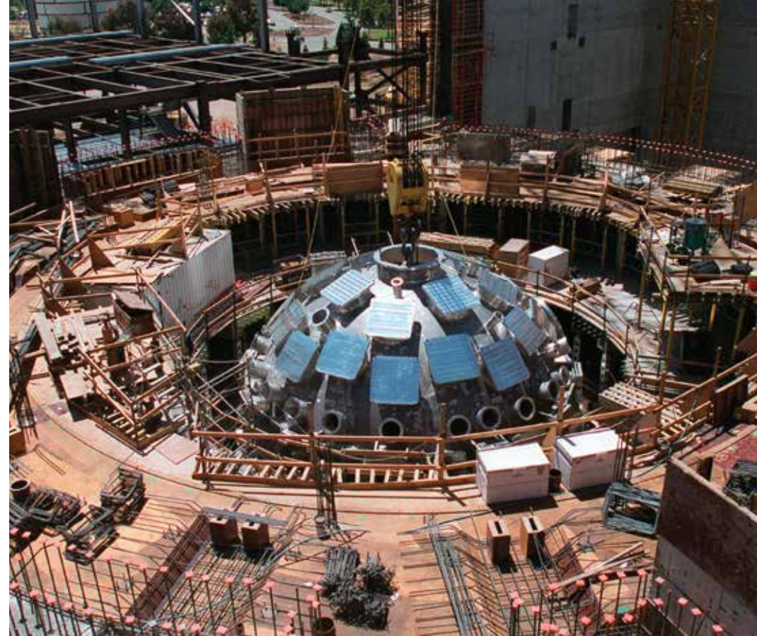
■ In June 1999, Manny the crane lifted the 287,000-pound, 10-meter-diameter NIF target chamber out of the steel tank in which it was constructed and into the NIF target bay. The NIF building was then completed around the chamber. Photos: LLNL
