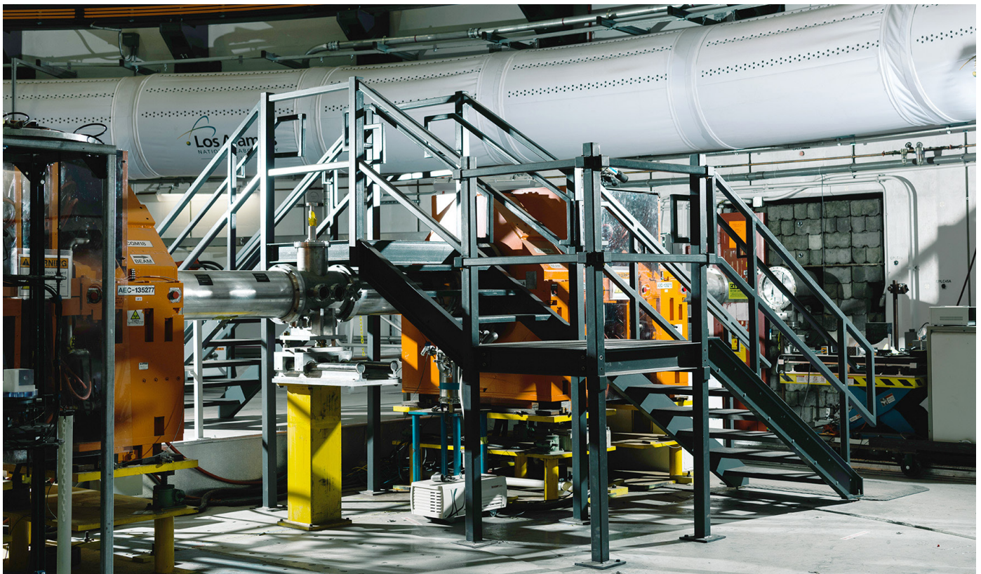
A new elevated walkway traverses the accelerator beamline, providing improved egress from the Proton Radiography Facility during the run cycle.
